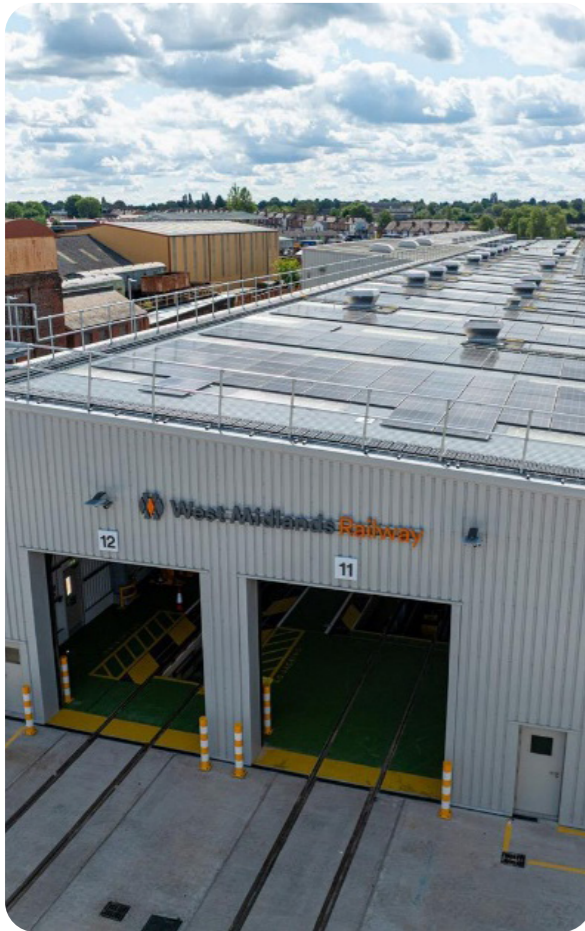
Tyseley Train Maintenance Depot Solar PV array
