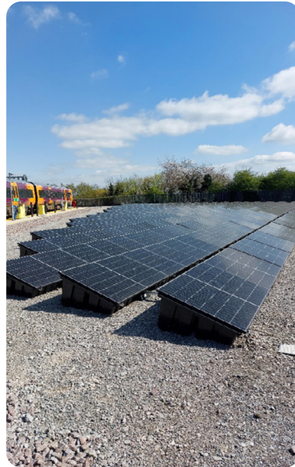
Bletchley Depot Solar PV array
